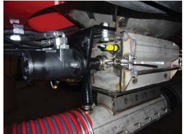
Hydraulic drive Meter Drive Motor
